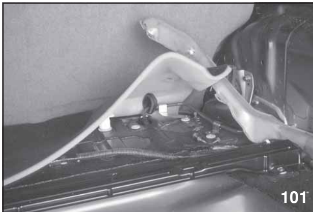
Vent Control Piping
